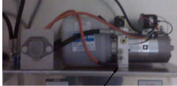
Tapped hole in pump frame marked GND
